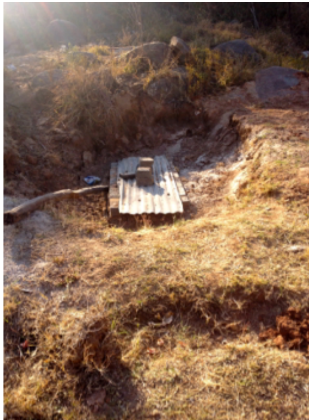
Unfinished toilet - mine CSR project, Segwaelane community
